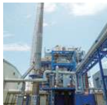
Biomass boiler, at REVACS Corporation
