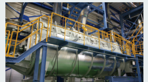
Cooker (Processes waste into biomass fuel in about 4 hours.)
